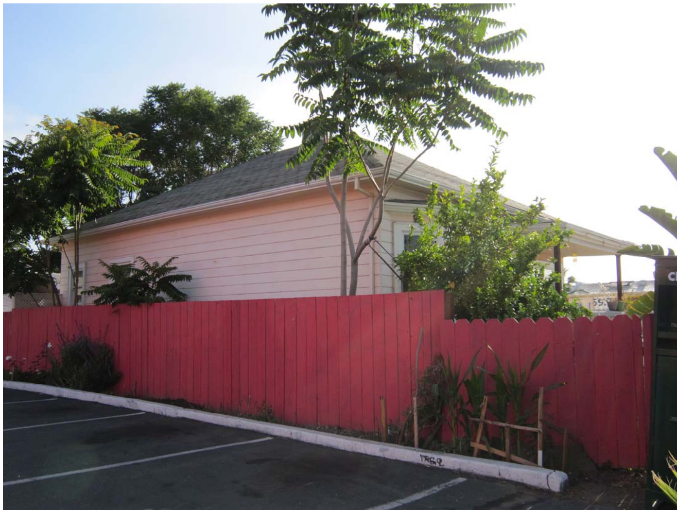
Photograph 3 815 W. San Carlos Street, San Jose View: West façade, the only window is in the infill rear porch area. Date: June 15, 2015
