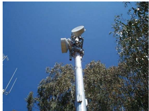
Emergency Communications Microwave Antennae at Eagle Rock
