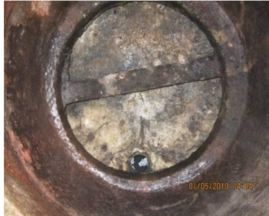
Submerged or Missing Baffle Wall Standpipe
