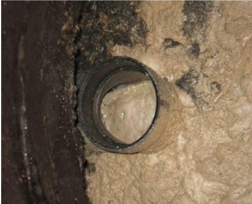
Grease in Effluent Standpipe
