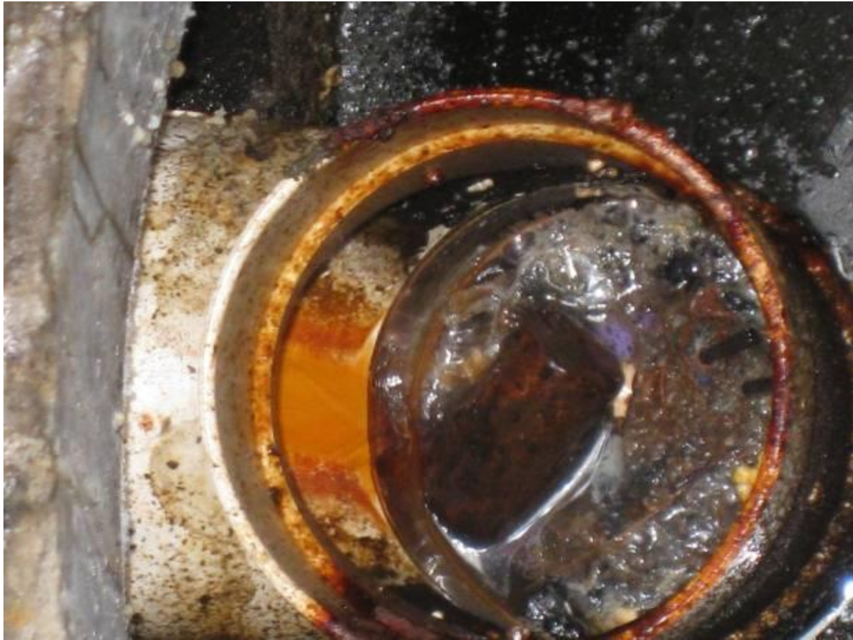
Debris Inside Inlet Standpipe
