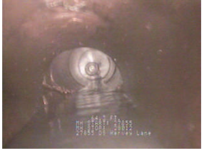
Broken and Offset at a Joint
