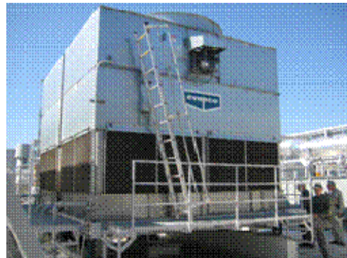
The cooling tower at the new Santa Clara County Crime Lab will use recycled water.
