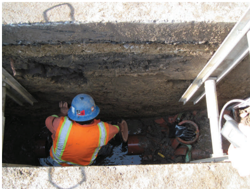
A point repair being performed to replace a broken sewer pipe at Vista Verde Drive.
