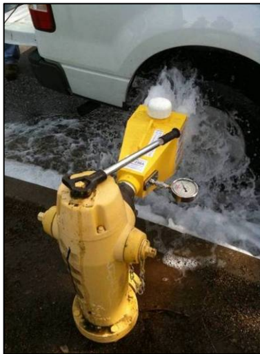
Potable water discharge
