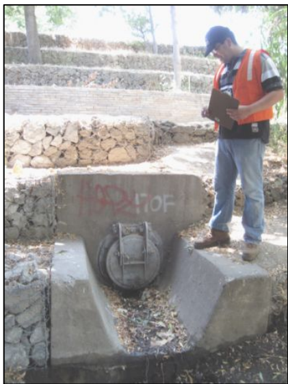
Collection System Screening
