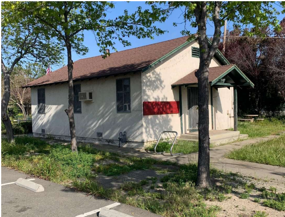
Figure 1. View of the building looking northwest from Liberty Street. The windows on the south façade are in their original locations and retain their original shape and size. Source: ESA, 2023.
