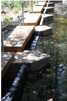
Flash Board Dam
