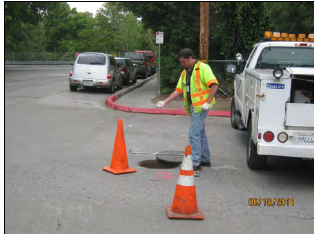
Environmental Inspector tracking down the source of a sanitary sewer leak into a storm sewer main
