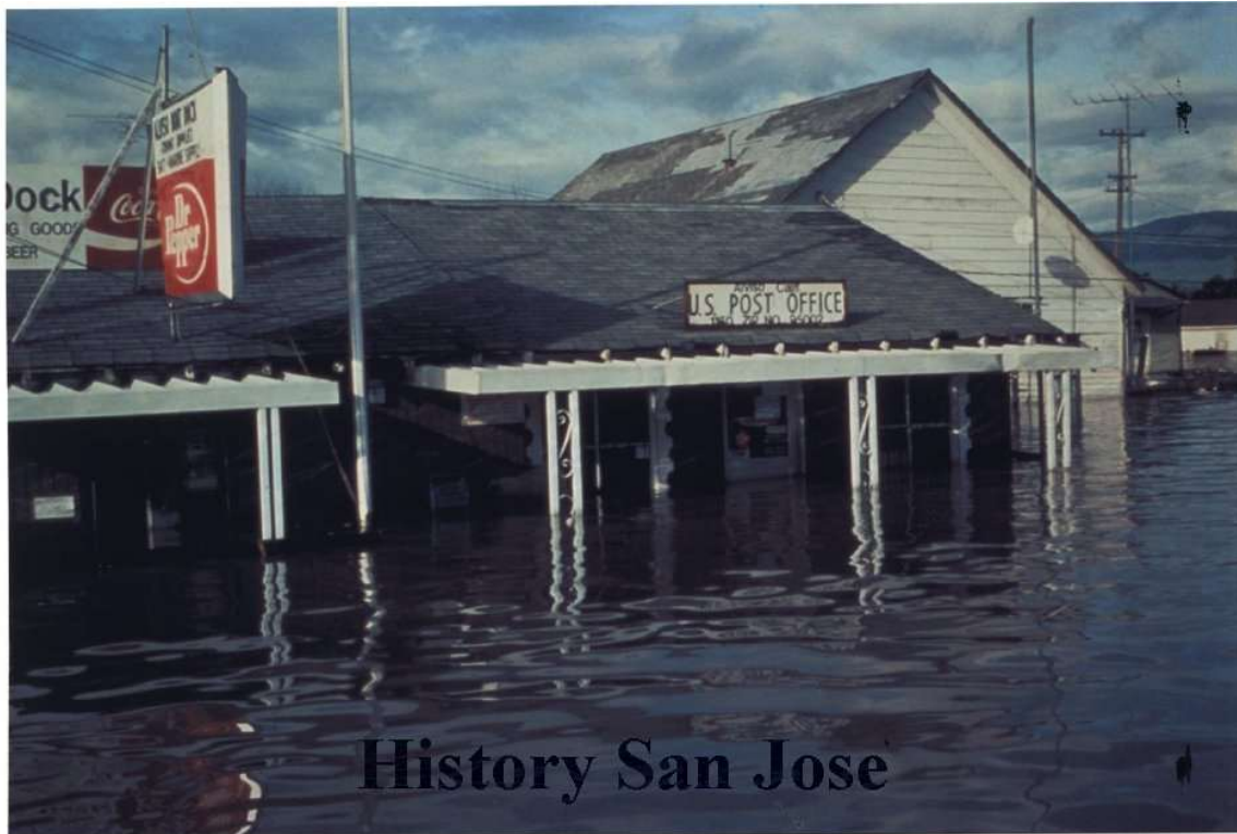
Figure 2: The subject building at 1160 North Taylor Street during the 1983 flood event. Photo courtesy of History San Jose ( https://historysanjose.pastperfectonline.com/photo/78E3C072-4E5B-4A99-8FBE-232348963738#gallery )
