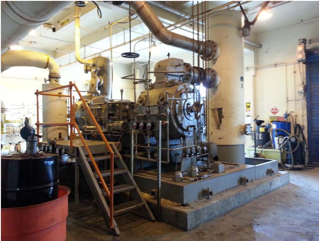
Figure 3: Existing Gas Compressor, GC4
