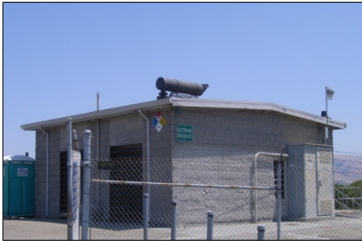
Gold Street Pump Station
