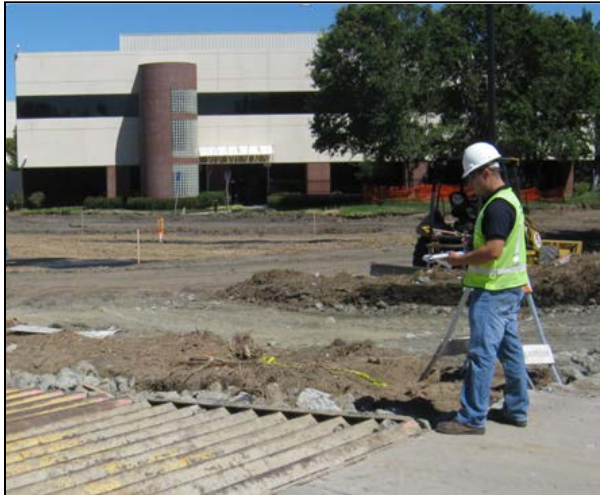
A City of San Jose Inspector checks the entrance/exit in the field
