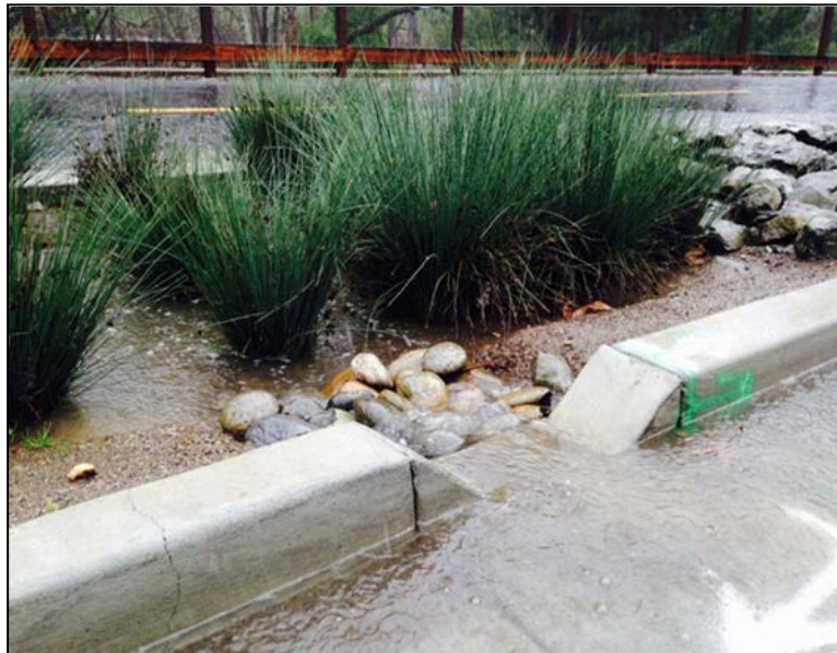
New and Redevelopment – stormwater runoff draining into bioretention cell through curb cut
