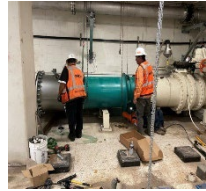
Fitting Spool on backwash piping
