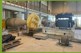
New motor installed on Secondary Blower #2
