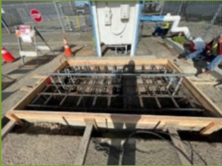
Storm Drain warehouse pump station
