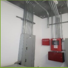
New fire panel for fiber connection
