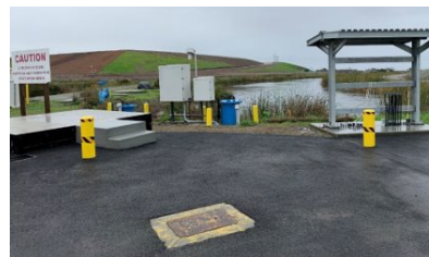
New ABB electrical panels under the canopy near the daylight station
