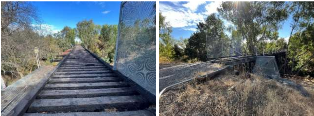
Figure 5. The south entrance of the trestle (left) and the north entrance of the trestle (right) (September 2022).
