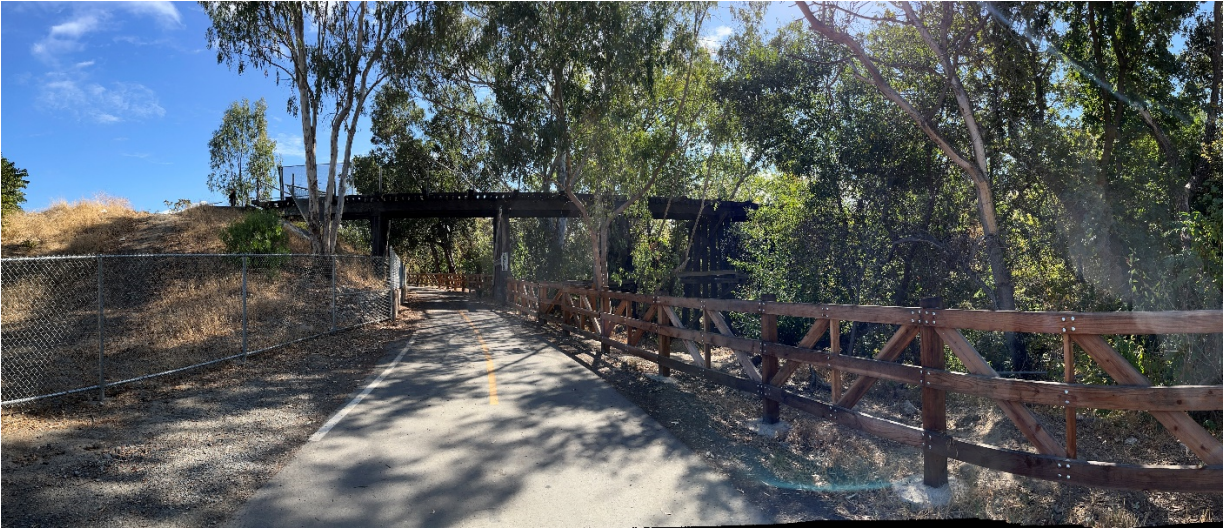
Figure 11. Looking east, a view of the Trestle from the Coyote Creek Trail with Coyote Creek on the bottom right (September 2022).
