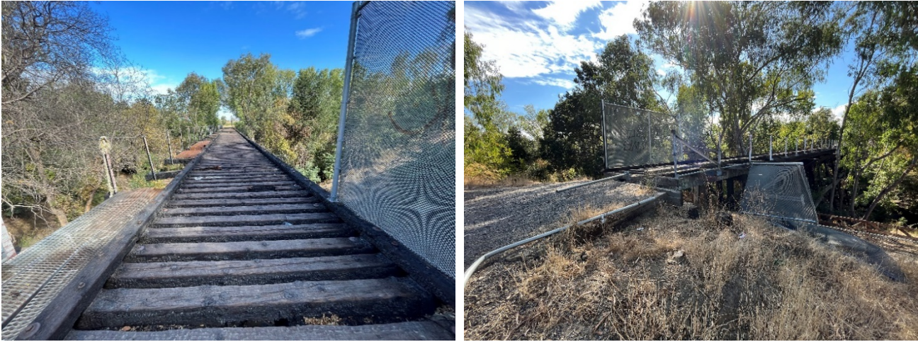
Figure 7. The south entrance of the Trestle (left) and the north entrance of the Trestle (right) (September 2022).
