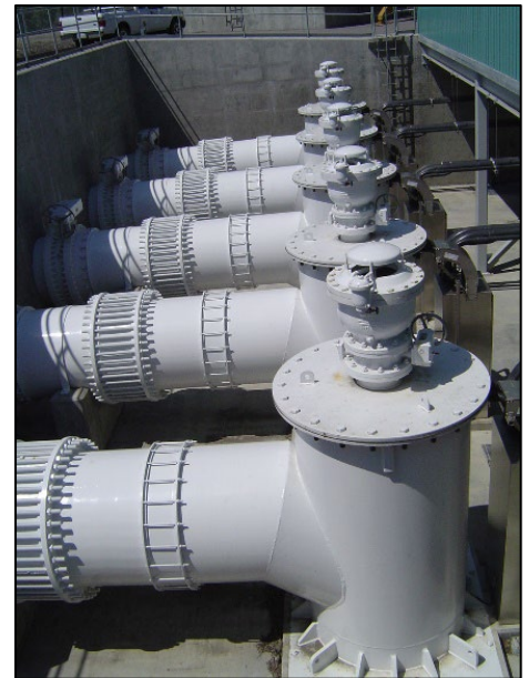
Pumps at the Rincon II municipally operated pump station
