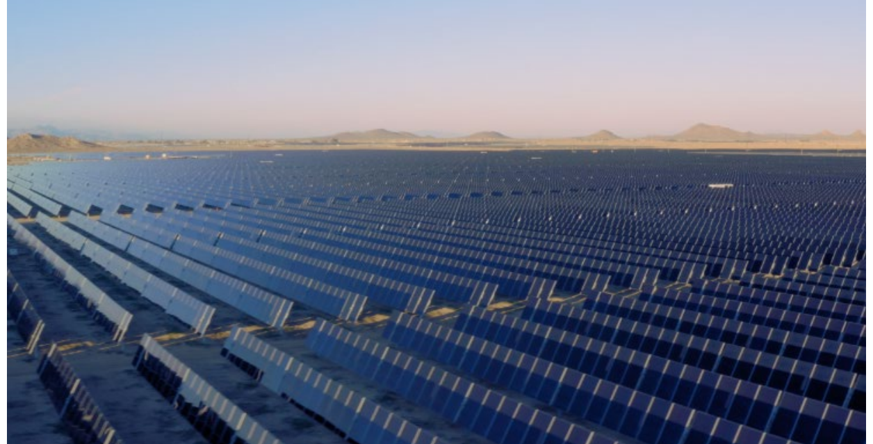
Solar field at SJCE's facility in Kern County
