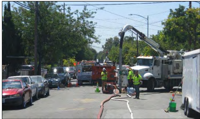
City Department of Transportation Staff working on a large sanitary sewer overflow (SSO)
