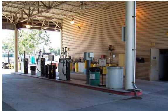
Figure 8: Examples of BMPs - Barrels of absorbent at fuel pumps
