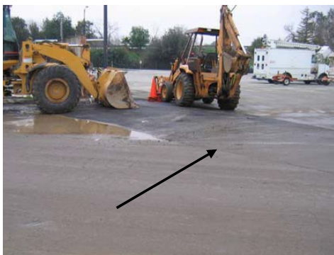
Figure 7: Black arrow points to the spill containment berm
