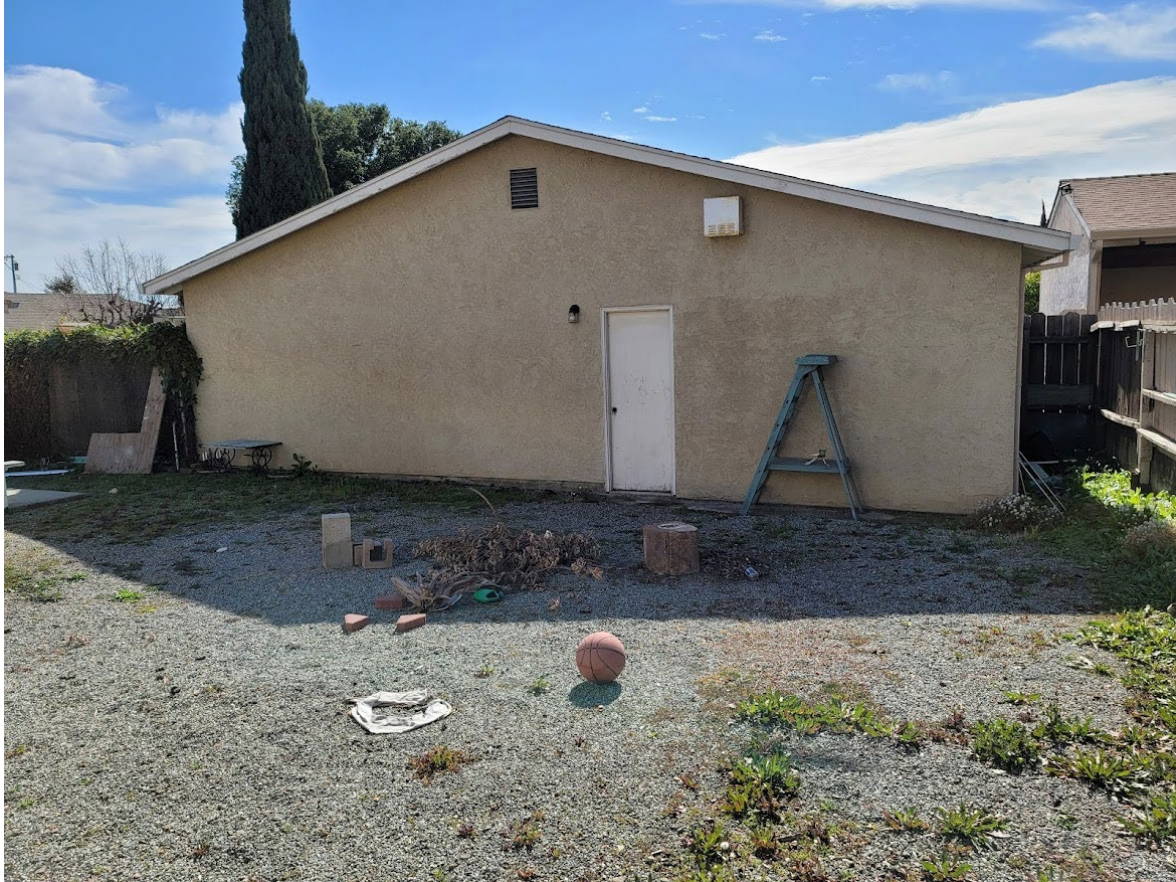
Photograph 6 125 Kirk Ave. San Jose- Garage View: East end, single doorway. Date February 19, 2022
