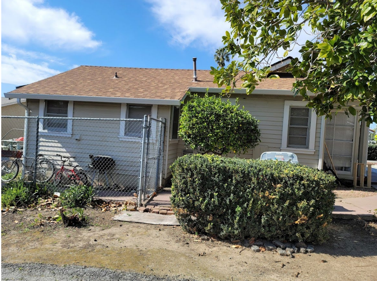
Photograph 2 125 Kirk Ave. San Jose View: South façade, note the extension of the side wall. Date February 19, 2022
