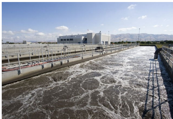
San José-Santa Clara Regional Wastewater Facility Aeration
