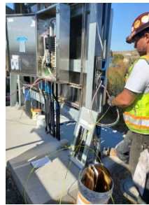
New ABB electrical panels under the canopy near the daylight station
