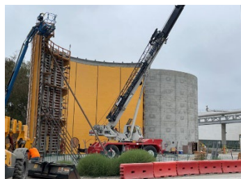
Sludge Storage Tank 2 forms and completed wall on Tank 1 to the right
