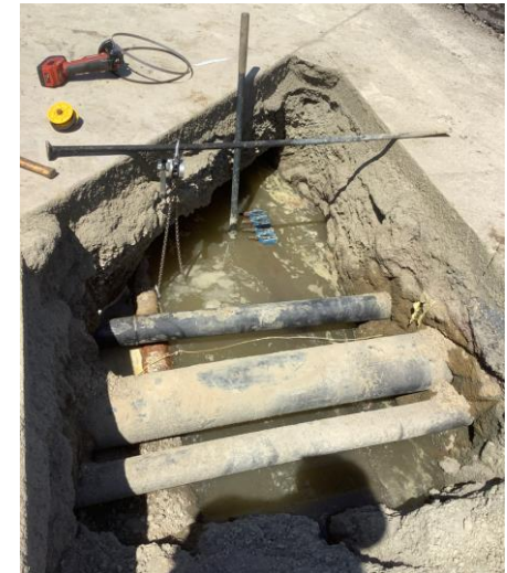
Pipeline Breaks and Repairs
