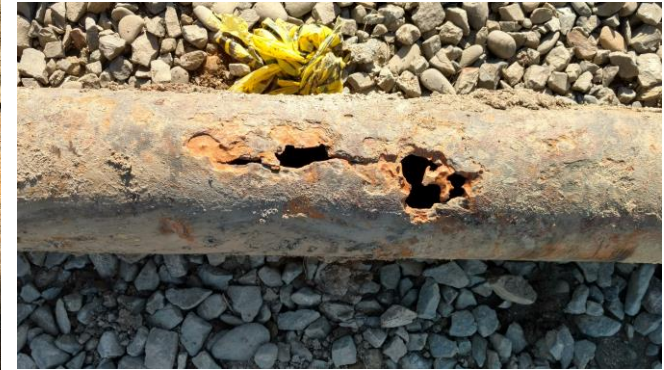
Pipeline and Valve Corrosion
