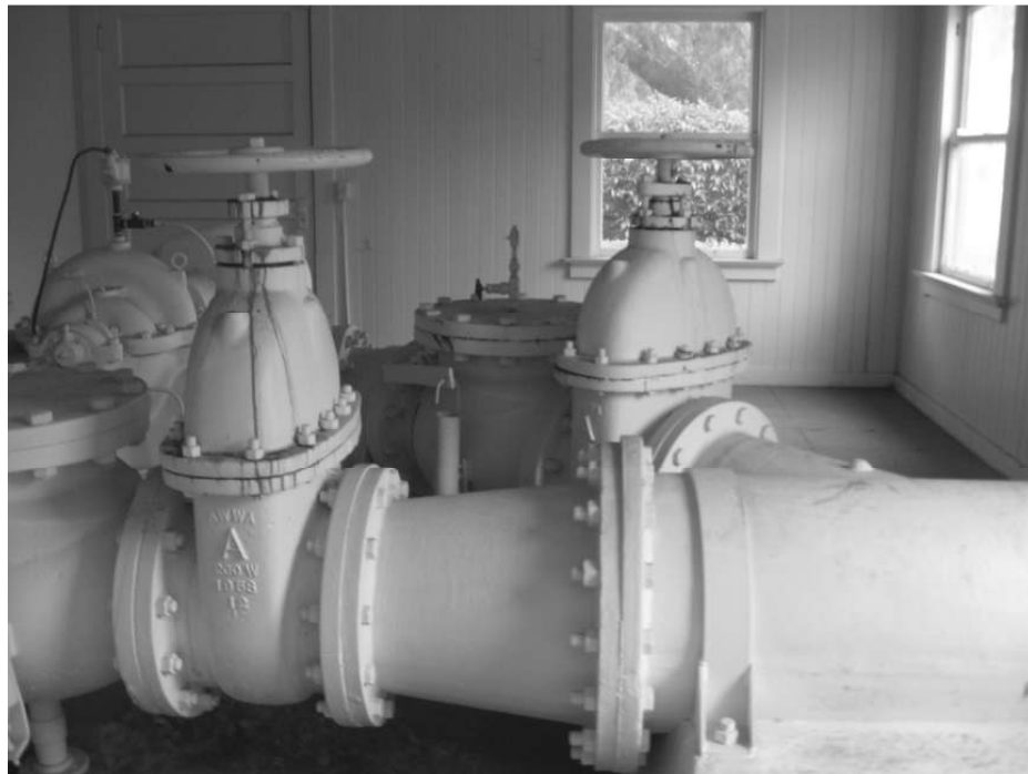
Photo 24: Interior view of pump and valve system.
