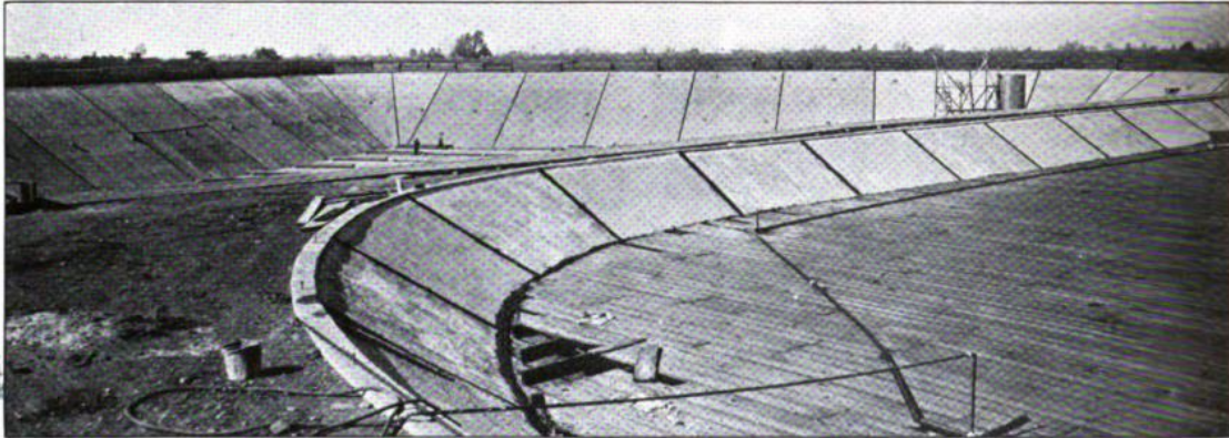
CAMBRIAN RESERVOIRS. NEW RESERVOIR IN BACKGROUND. OLD RESERVOIR IN FOREGROUND DURING RECONSTRUCTION BEFORE OLD ROOF WAS REMOVED
