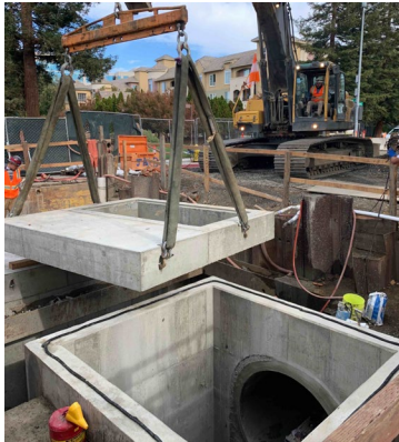
Top of Precast PCC vault
