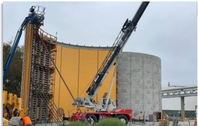
New sludge storage tanks
