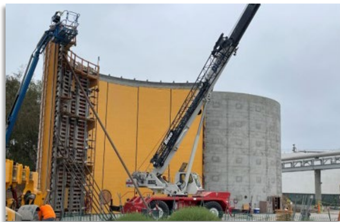
New sludge storage tanks
