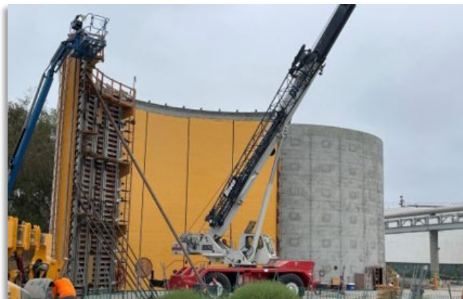
New sludge storage tanks
