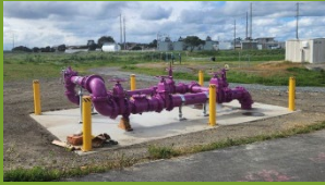
Newly installed SBW Flow Meter and Backflow Preventer
