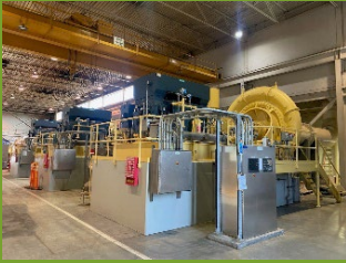
Process Aeration Blowers with improvements
