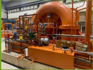
Tertiary Blower Building with improvements
