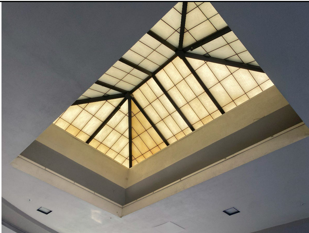
7. This photo depicts a concave panel section overhanging Good Samaritan Emergency Department.
