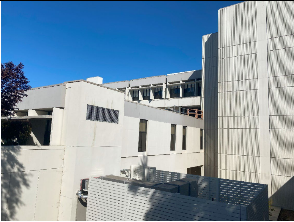
10. This photo depicts another section of the main hospital building's exterior, with a vent on the lefthand side.
