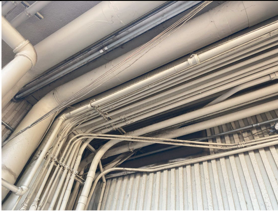
6. This photo depicts piping running along the exterior of the hospital building.
