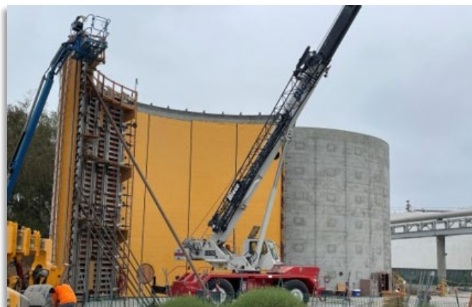
New sludge storage tanks
