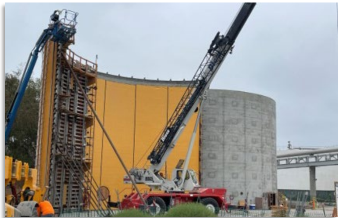
New sludge storage tanks
