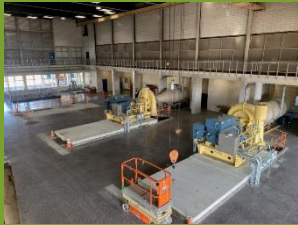
Secondary Blower Building with improvements
