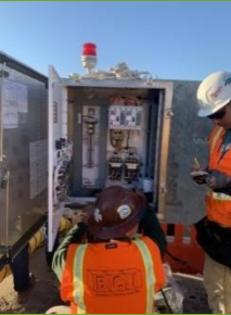
Power station testing
