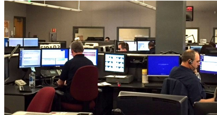
Image of SJPD Communications Center Control Room. Source: SJPD
