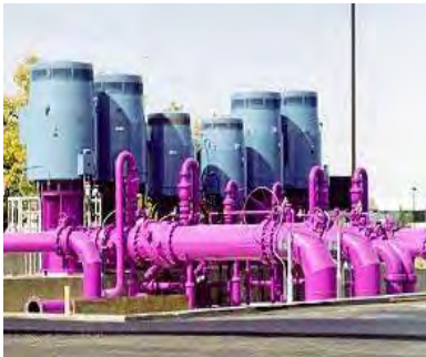
Purple pipes supply about 0.2 million gallons per day of recycled water.
