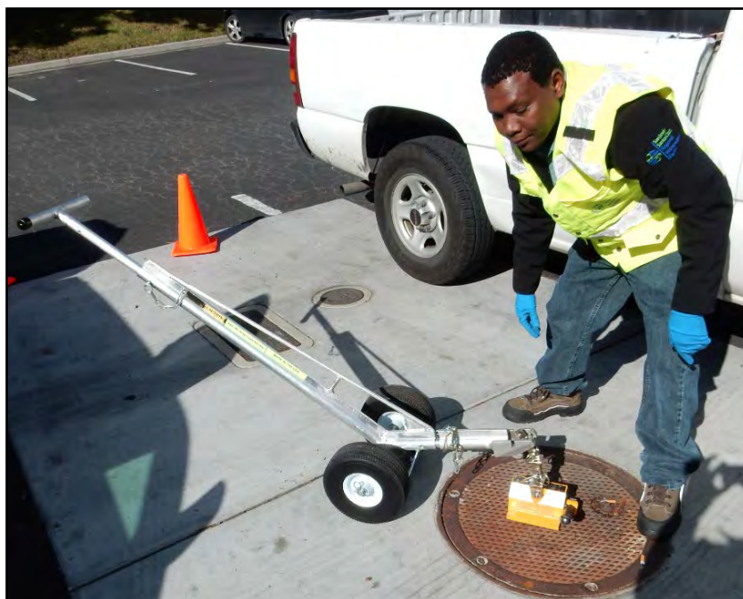
Inspector Mahmoud Jillo lifting the cover off a restaurant interceptor.
