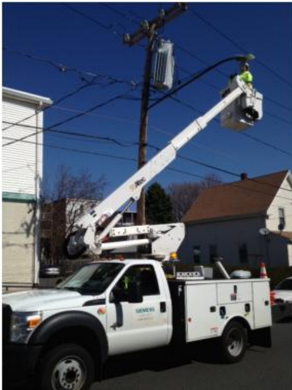
Siemens crews use the “Think Safety” motto to deliver the retrofit of over 10,000 streetlights without a single safety incident.
