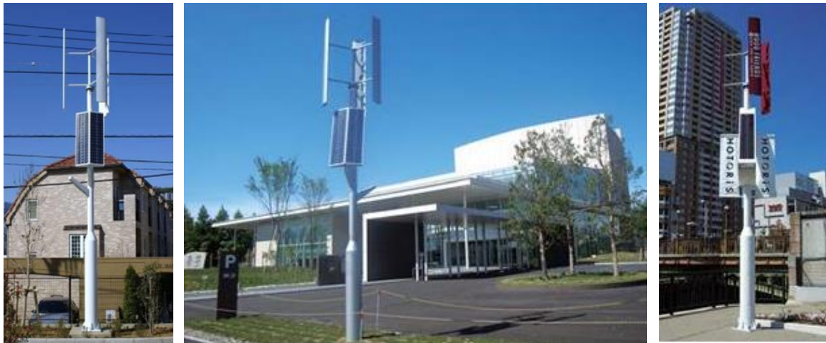
Figure 8: Installation of solar and wind power generation station on a pole in various city locations – residential, civic center, and commercial area (from left to right)
