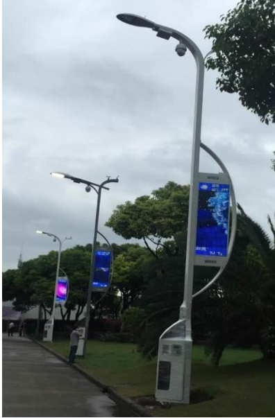
Figure 9: A Smart Light Pole with LED “Banner”
