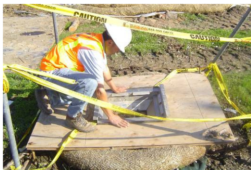
Contractor installing protective BMPs around a storm drain inlet at the Edenvale Community Center
