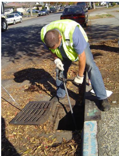
Department of Transportation Maintenance Worker services a catch basin on El Dori Drive
