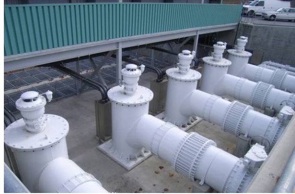
Pumps at the Rincon II pump station
