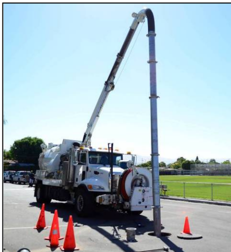
Vactor truck preparing to clean out HDS unit located at Bulldog Boulevard.
