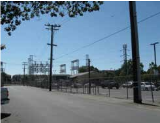
11) PG&E Substation on Proposed Stadium Site
