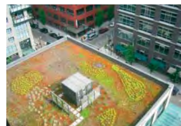
Green roofs improve water retention and indoor climate, and make the roofscape visually attractive.
