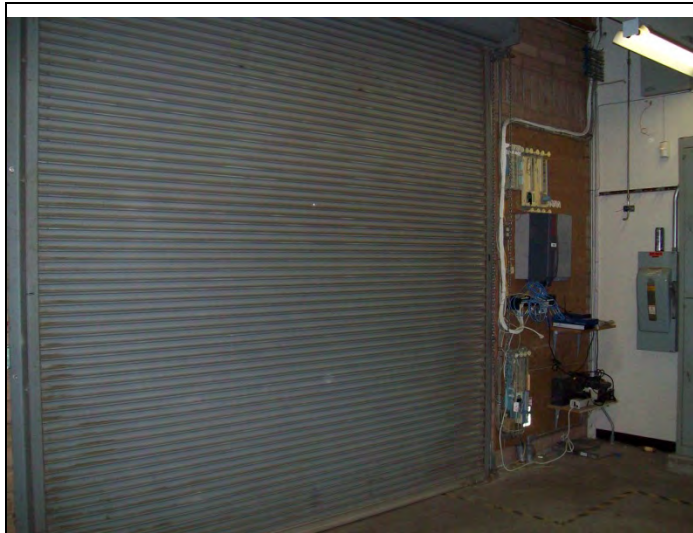
Photo No: 19 Picture Direction: Interior Description: Grade level roll-up door in maintenance bay.
