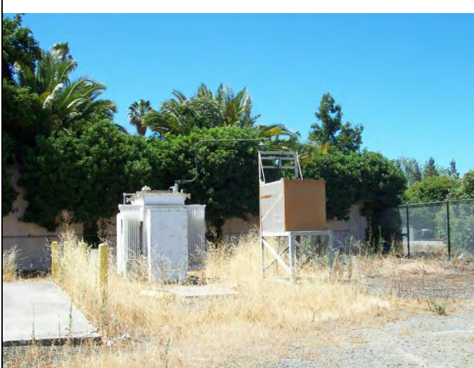
Photo No: 13 Picture Direction: SSE Description: Plant transformer in southwest portion of backyard.
