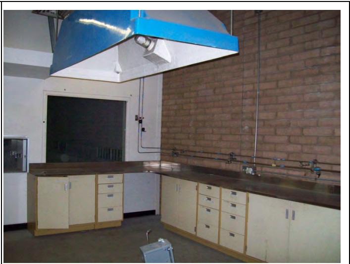
Photo No: 20 Picture Direction: Interior Description: Maintenance bay area near air shower room.
