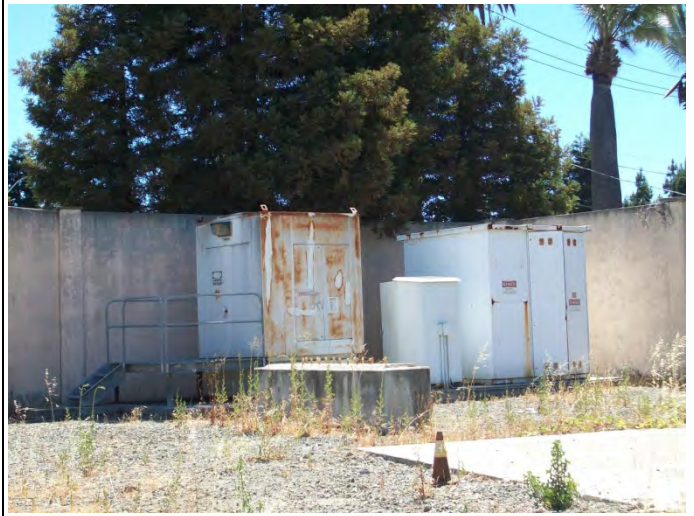
Photo No: 14 Picture Direction: SW Description: Incoming power from PG&E for plant transformer in southeast portion of backyard.
