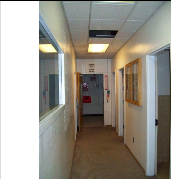
Photo No: 18 Picture Direction: Interior Description: Hallway inside Property building; typical interior space.
