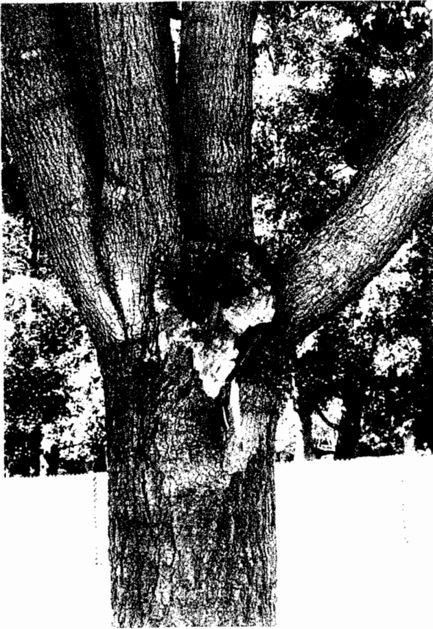
Trees # 775 Callery pear – broken limb as a result of attachment at an acute angle- virtually every Callery pear on site has this problem of varying degree
