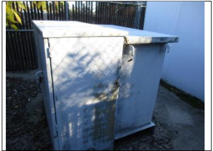
16. View of a pad-mounted transformer in the equipment enclosure adjacent to the west
