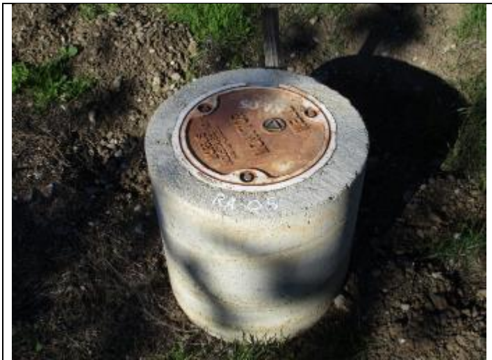
5. View of a groundwater monitoring well RA-05 along the southern property line
