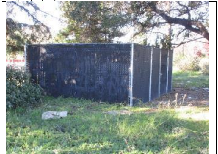
12. View of groundwater remediation equipment in enclosure adjacent to the west
