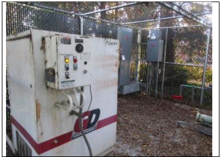
14. View of groundwater remediation equipment in the enclosure
