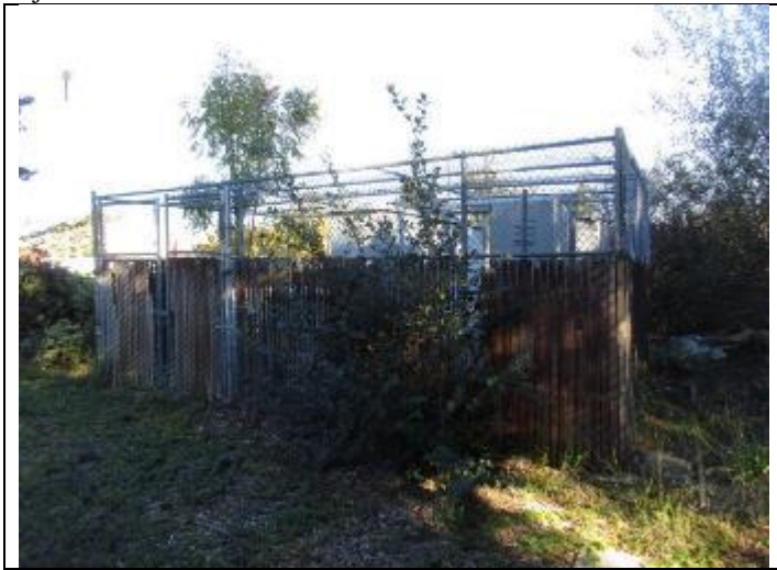
15. View of electrical equipment enclosure adjacent to the west
